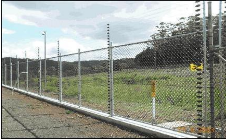
Figure 2: Electric Power Fence inside Chain Wire Mesh Fence
