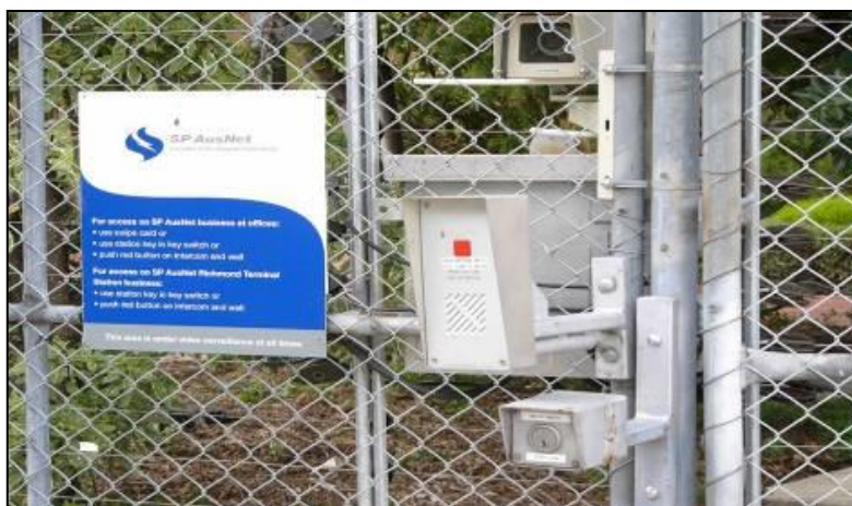
Figure 5: Electronic Access Control, User Interface
