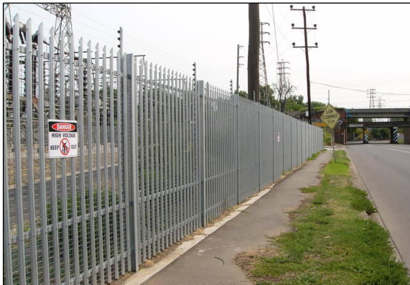
Figure 1: Palisade Security Panel with Concrete Plinth and electric power fence
