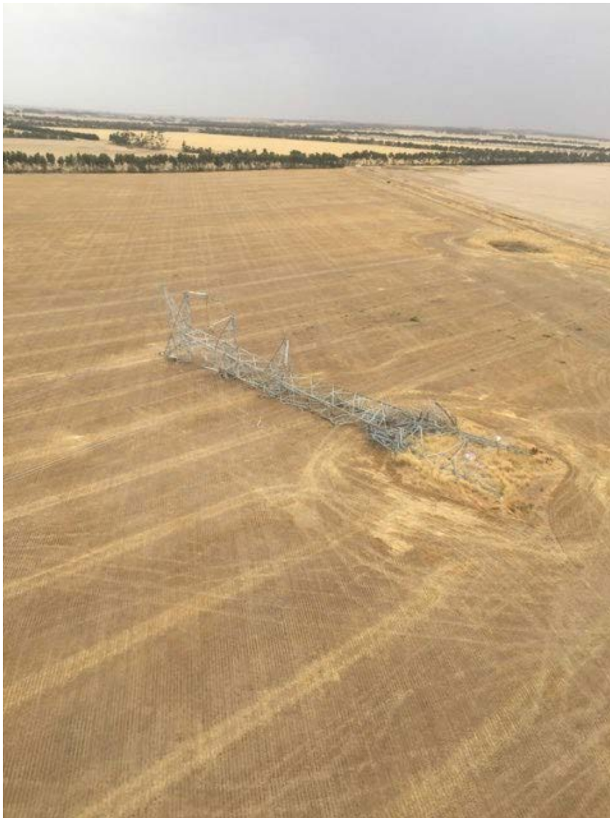
Figure 2: One of the collapsed 500kV double circuit towers
