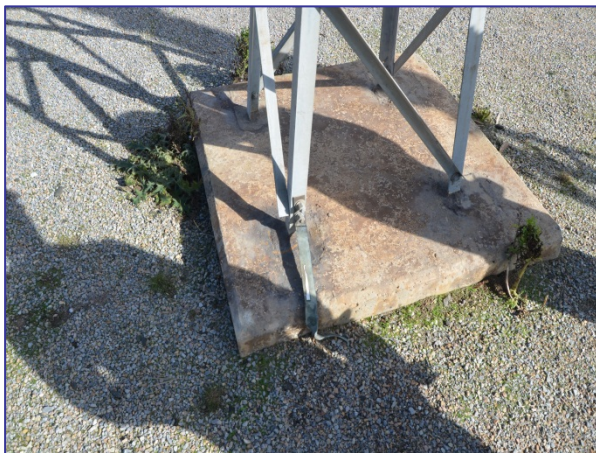
Figure 5 – Damaged earthing conductor
