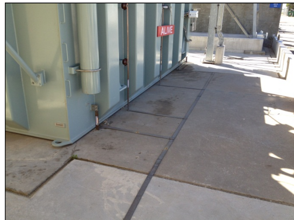
Figure 2 – Copper flat earthing conductors
