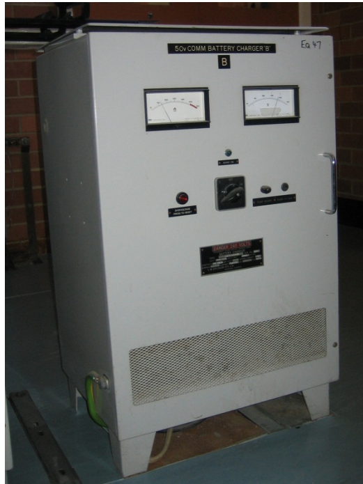
Figure 4 – 48V Battery Charger at KTS
