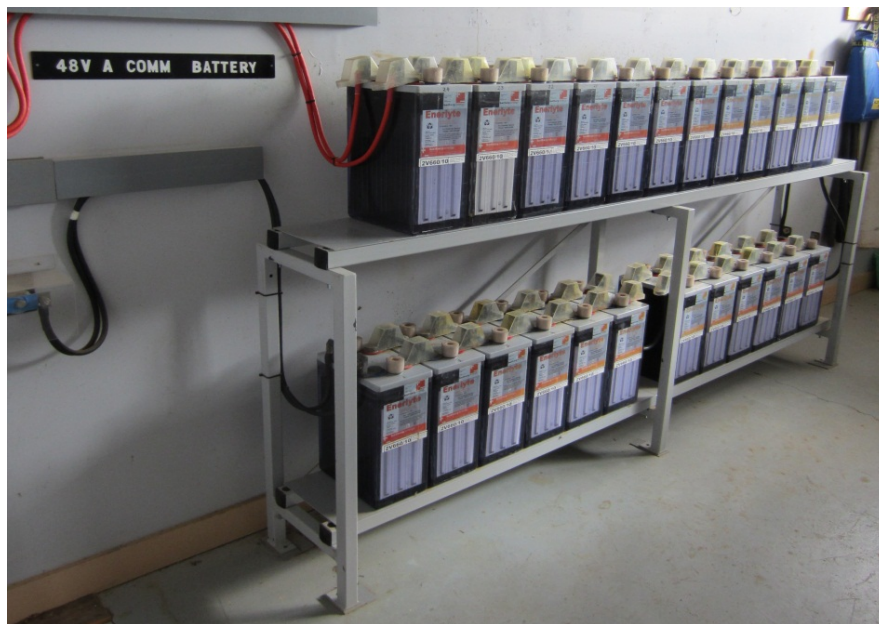
Figure 1 – Standard 48V Battery Bank of 2V Cells
