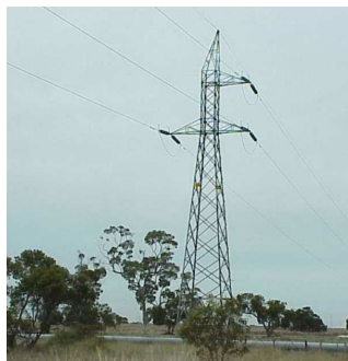
F1836 Tower Tension Structure (26).
