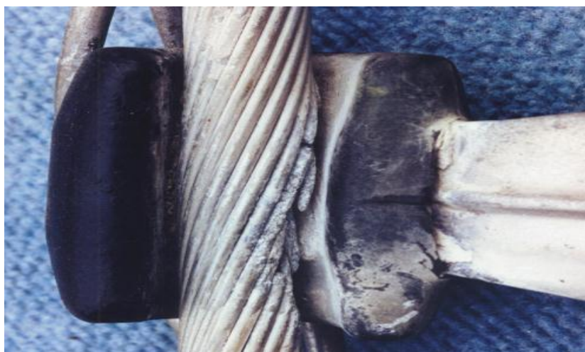
Image 1. Severe ES2 Damper Damage
