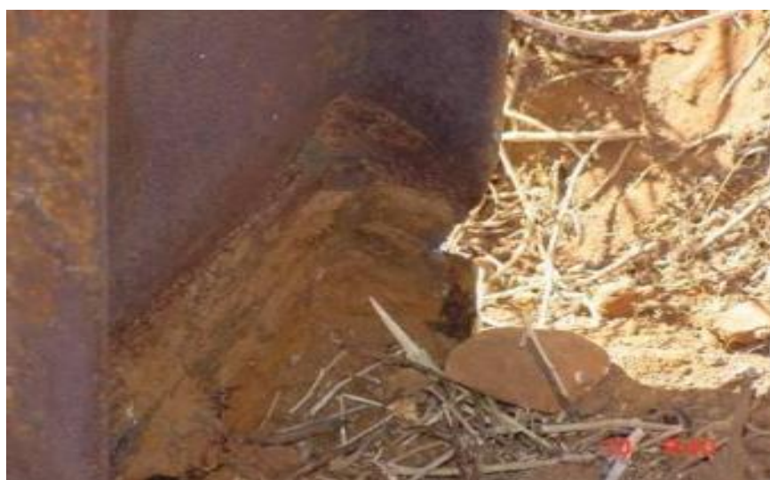
Image 6. Stobie Pole – Ground Line Corrosion
