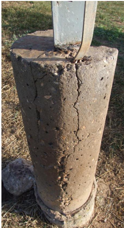
Image 7. Unreinforced and (Exposed) Foundation
