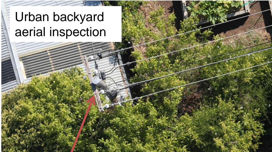
Crossarm defect detected through aerial inspection
