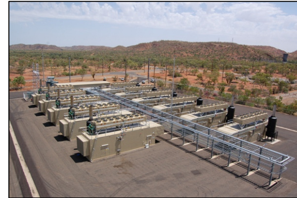
X41 Power Station, Mt Isa - EII
