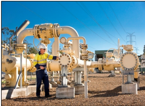
Ellengrove Gate Station – gas from Roma Brisbane Pipeline enters APT Allgas Network
