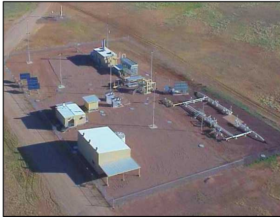
Morney Tank Compressor Station
