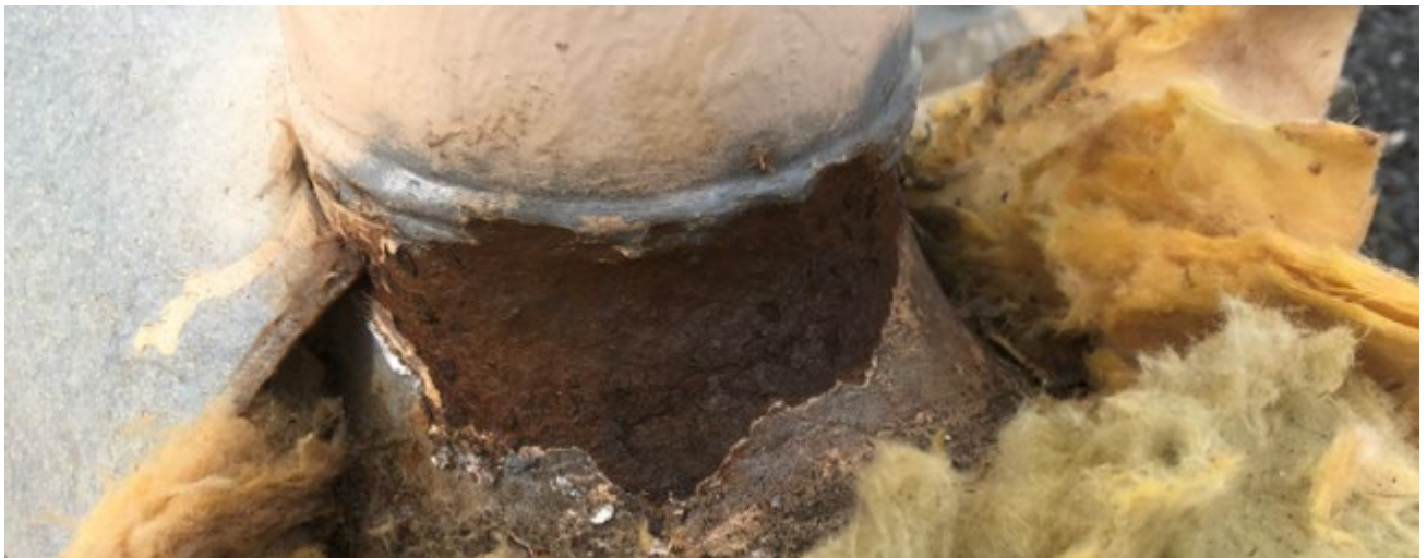
Cladding and insulation partially removed (from above photo) showing coating failure and active corrosion requiring repair.
