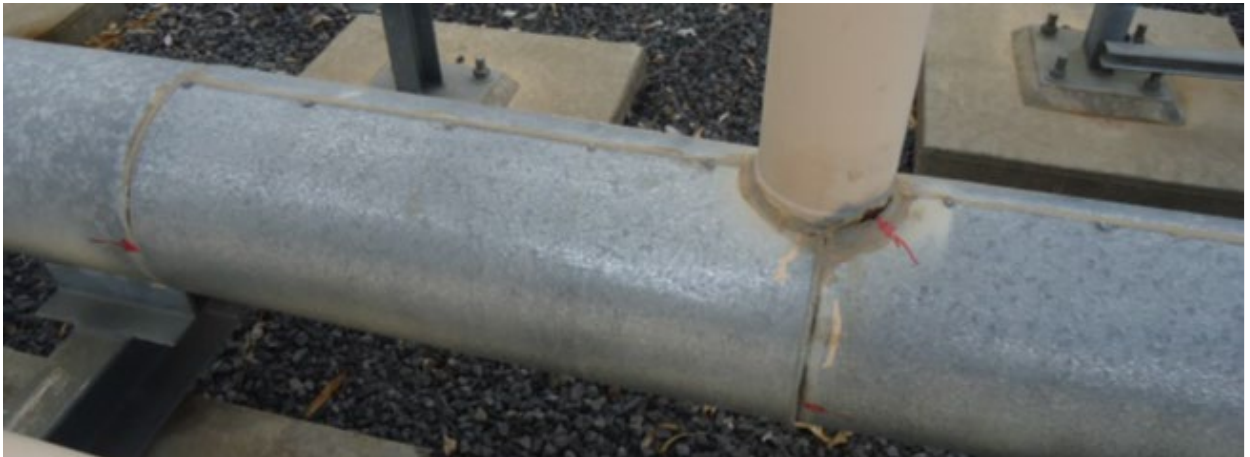
Insulation / cladding failure showing water ingress point.
