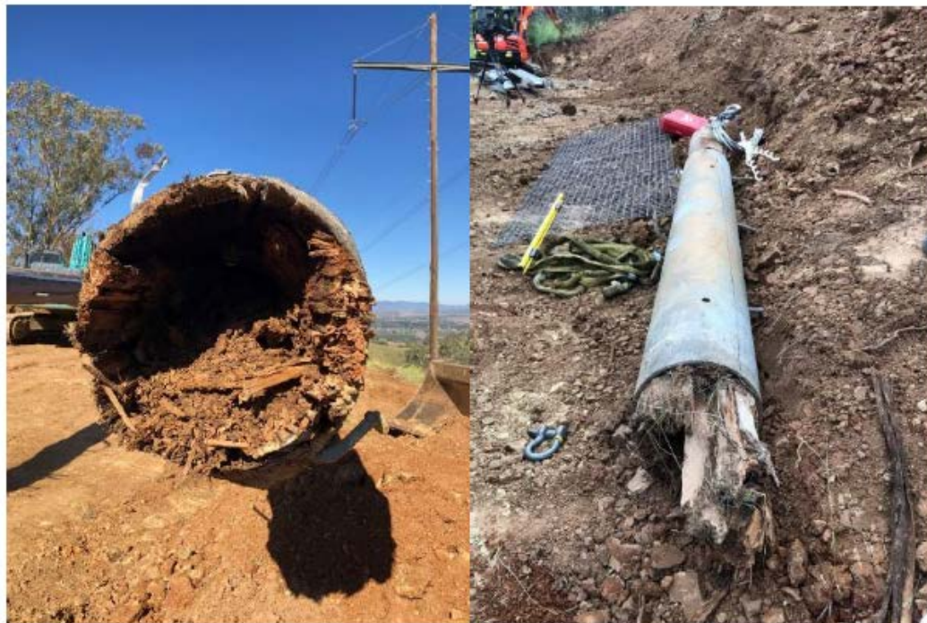
Figure 3.2: Example of wood rot on Line 86
