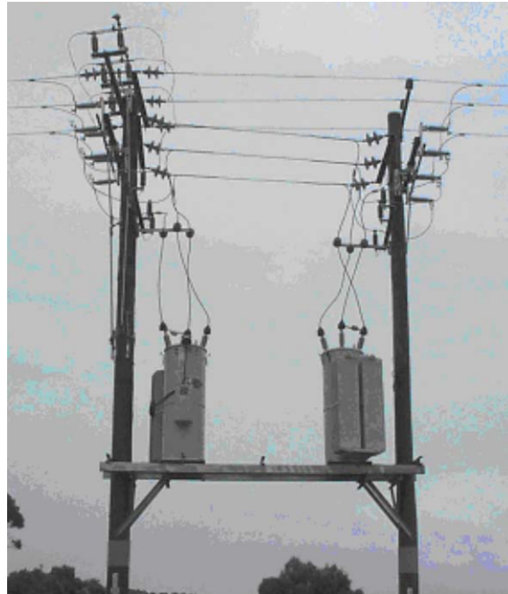
Figure 2: Typical Pole-Mounted Single Phase Open-Delta Regulator
