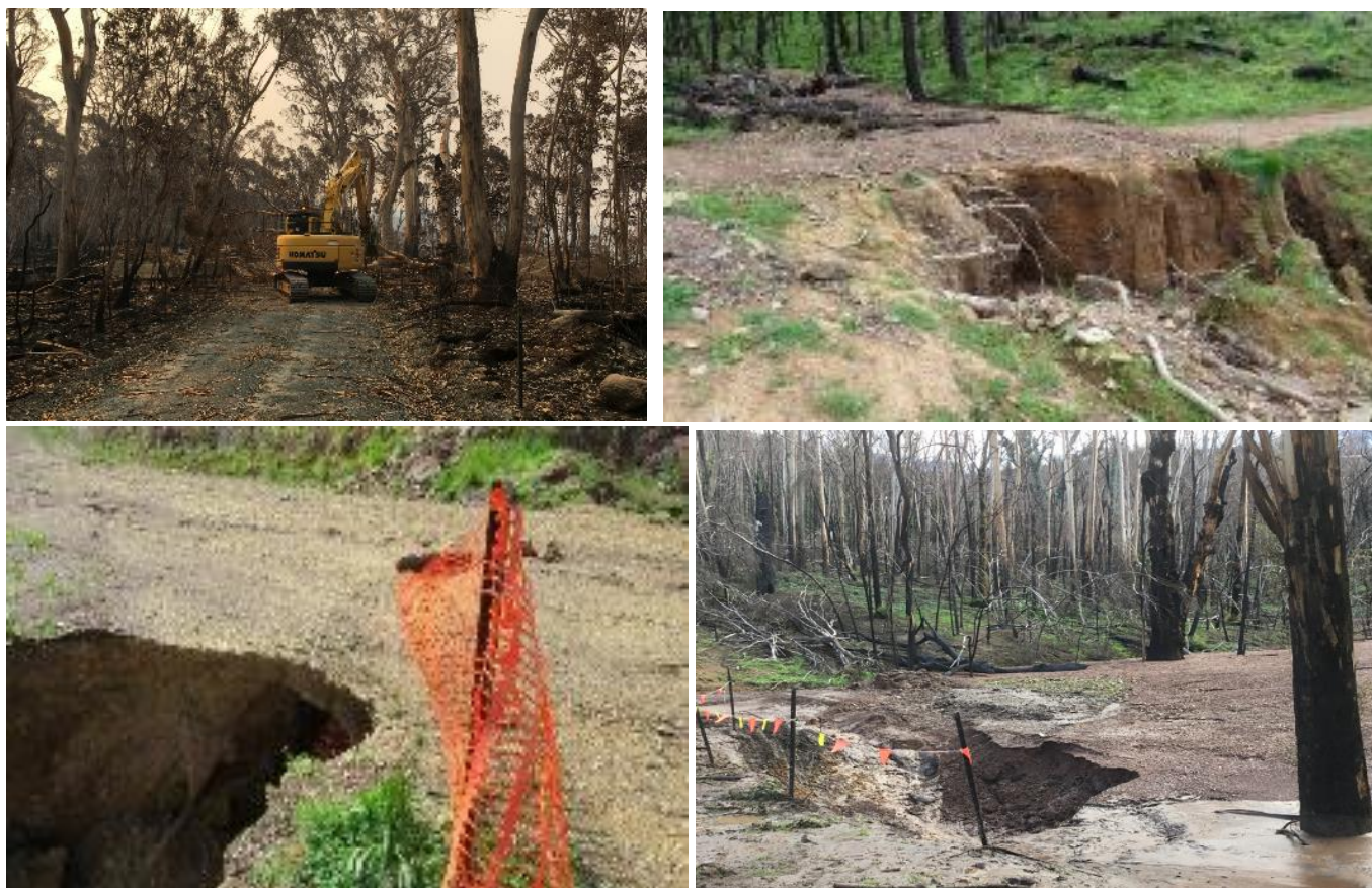
Figures 7 – Examples of damaged vegetation and access tracks
