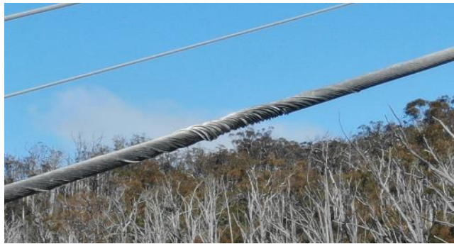
█, RHS PHz Conductor Fire Damage
