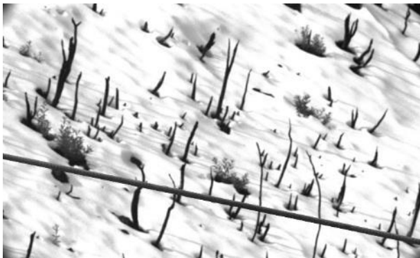
Span 8 (Caging & bulging conductor)
