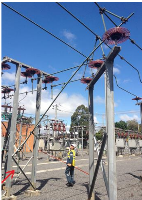
Figure 4–17: Failed Pin and Cap Insulator
