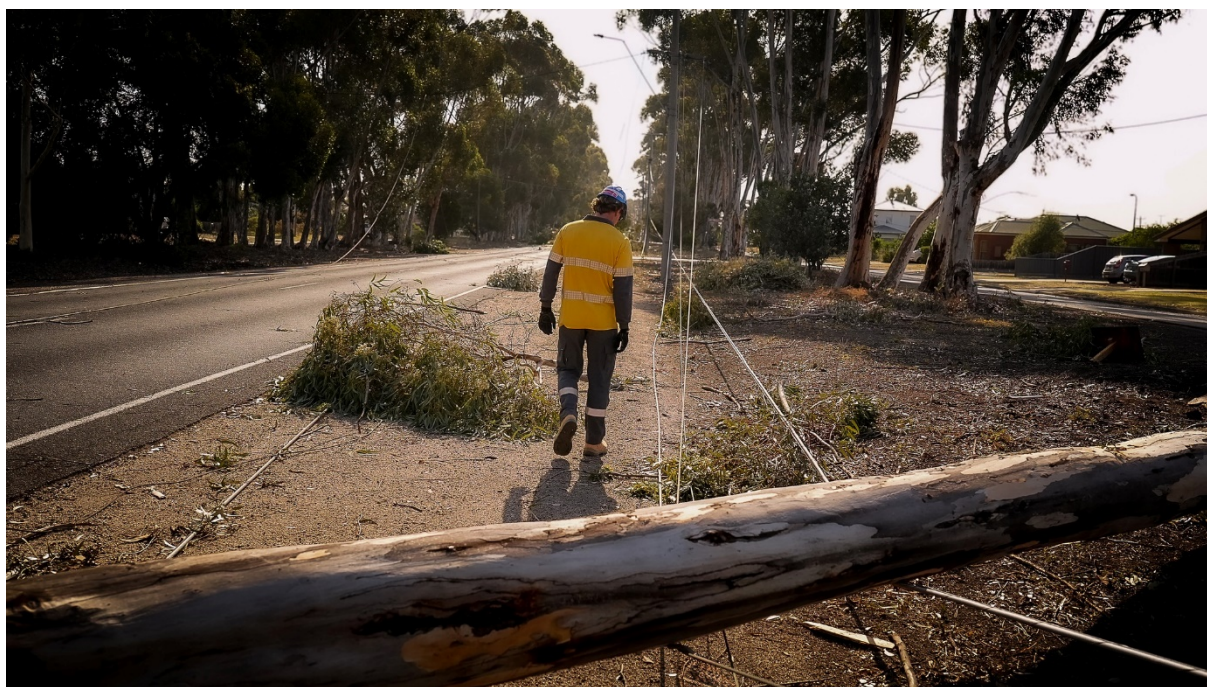
Note: Powercor lineworkers restoring supply in Lara following major storm damage in February 2024
