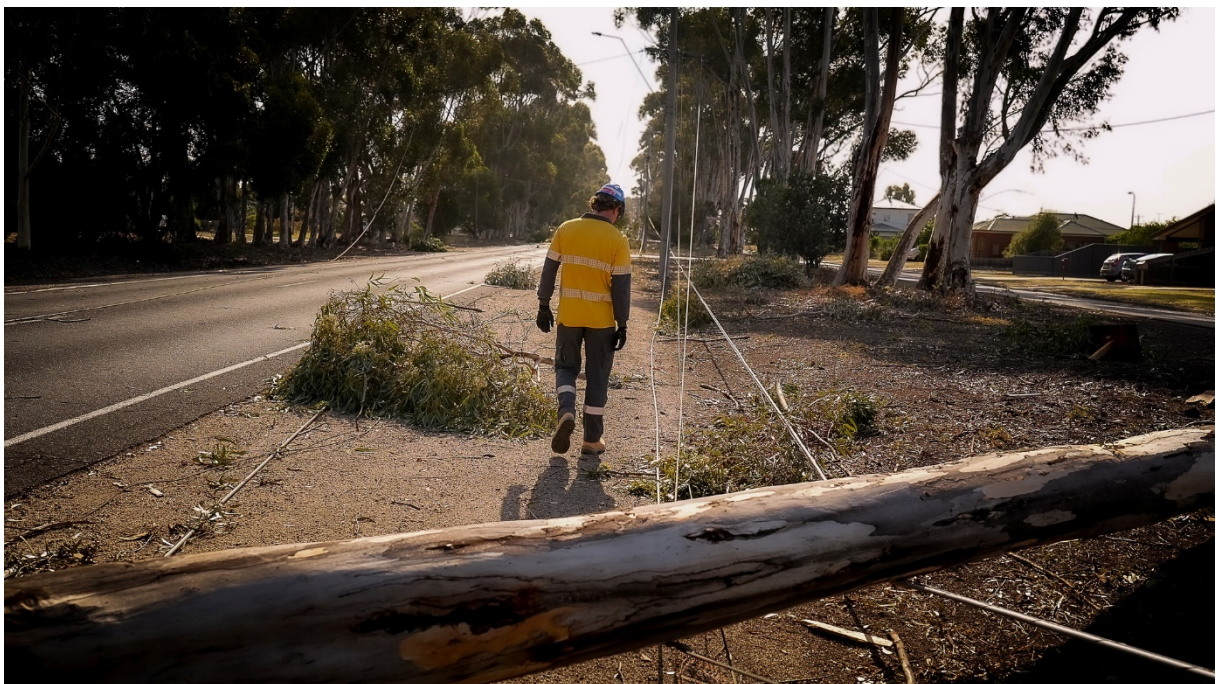
Note: Powercor lineworkers restoring supply in Lara following major storm damage in February 2024
