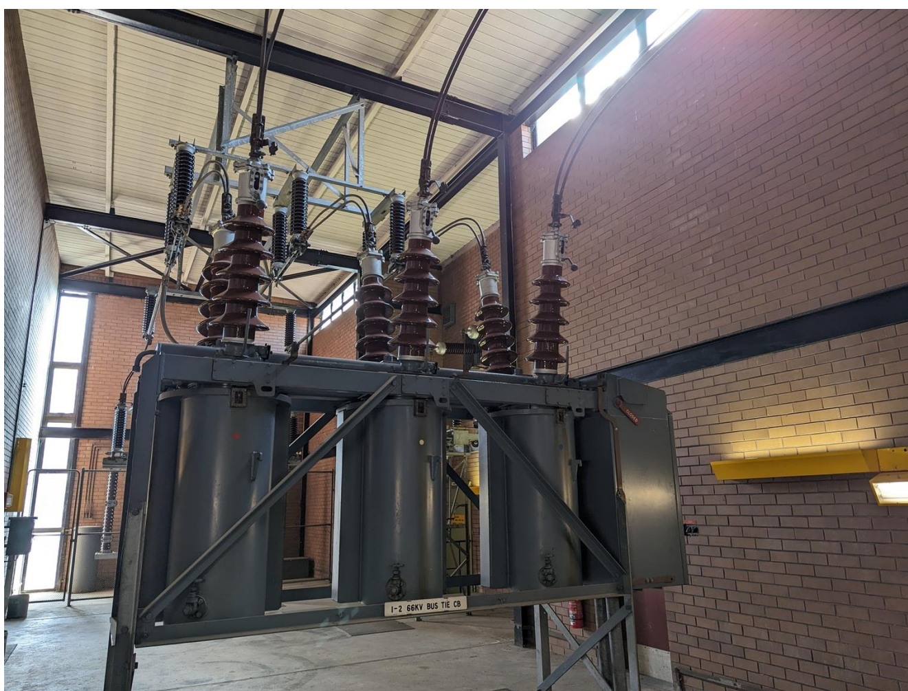
Figure 2-2: NH 1-2 66kV Bus Tie CB
