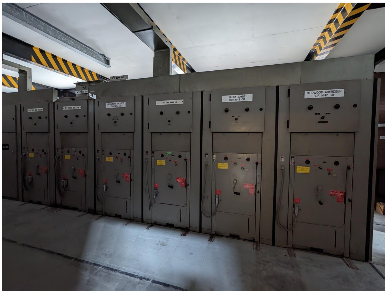
Figure 2-3: NH No.1 22kV Switchgear
