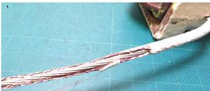
Image 2. Deteriorated consumers mains wiring
