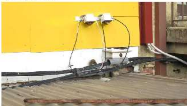
Image 1. LV ABC contacting roof and in close proximity to deteriorated consumer mains cable
