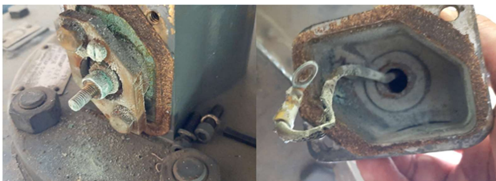
Figure 2-5 Damaged Tap Set and Secondary Wiring
