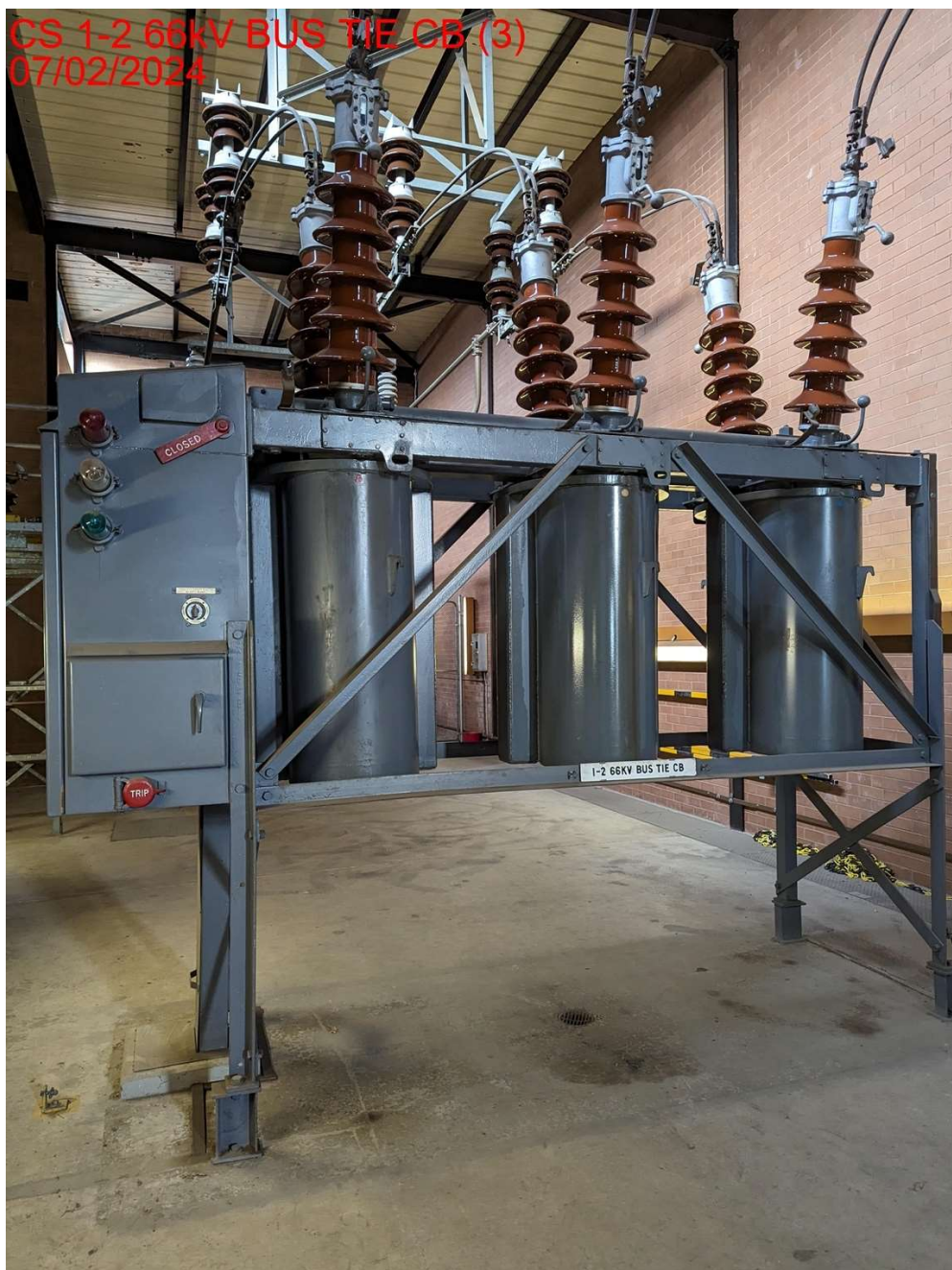
Figure 2-2: CS 1-2 66kV Bus Tie CB
