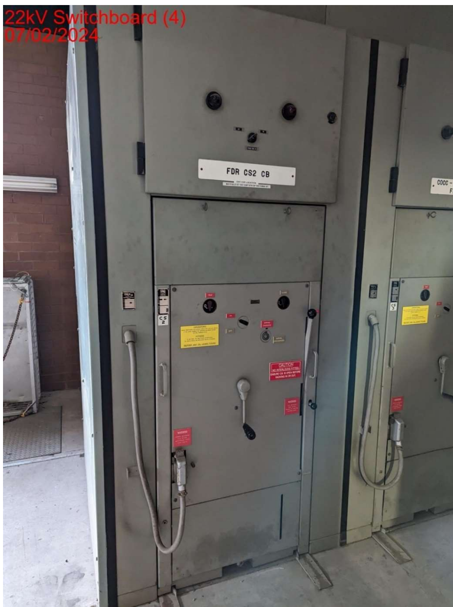
Figure 2-3: CS 22kV Switchgear
