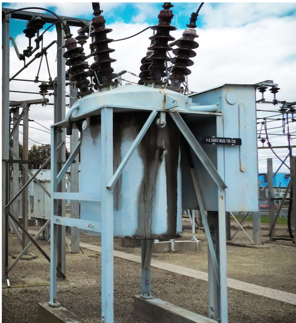
Figure 2-3: CN 22kV Switchgear
