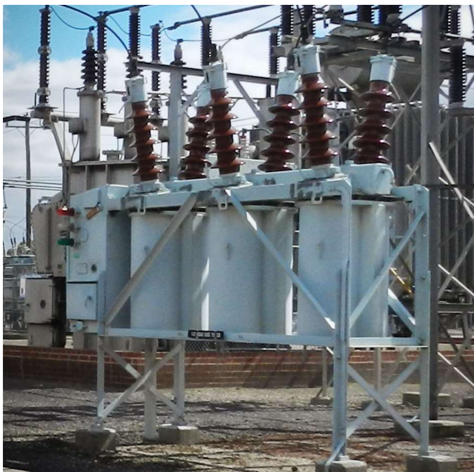
Figure 2-2: CN 1-2 66kV Bus Tie CB
