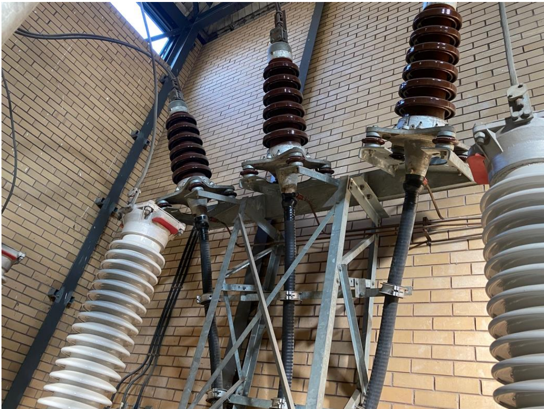
Figure 2-2 66kV ST Oil Filled Feeder Exit Cable at Newport (NT) Zone Substation (BLTS Feeder)
