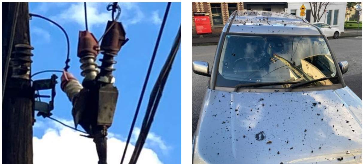
FIGURE 9 FAILED BOX TERMINATION AND PITCH SPLATTER FROM FAILURE
