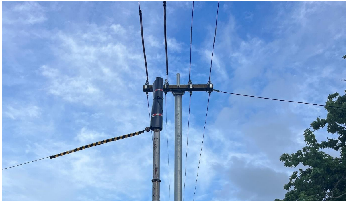
FIGURE 2 NEW YARRA TRAMS POLE WITH OUR ASSETS AND OLD YARRA TRAMS POLE
