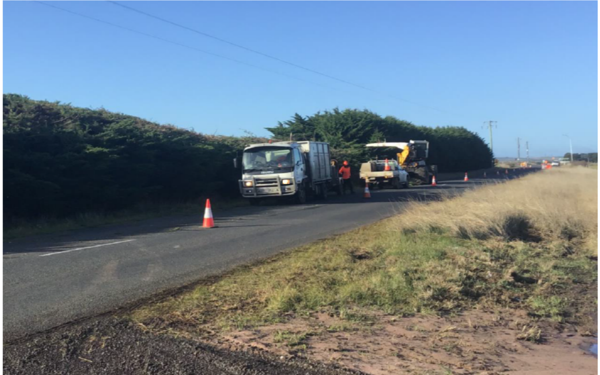
Significant volume of vegetation being removed from cypress hedge using all terrain Jarraff - Geelong zone substation
