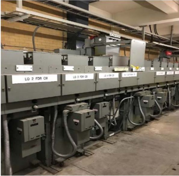
Existing Email HQ compound filled double bus switch board - Bus A shown
