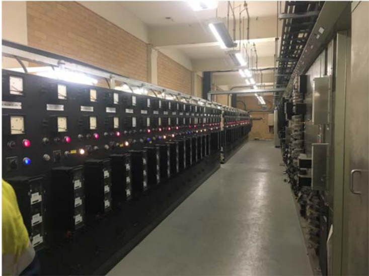
Existing early 1970's electromechanical protection relays
