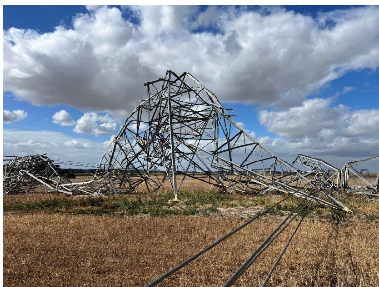
Figure 3: Transmission Towers on the Moorabool to Sydenham (MLTS-SYTS) 500kV No 1 and No 2 lines collapsed, resulting in the loss of those lines.
