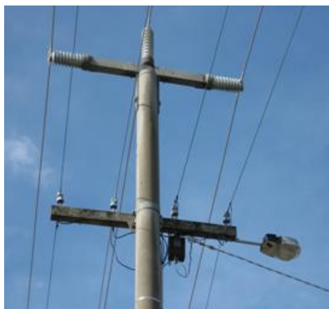
Figure 3 – Typical Concrete Pole
