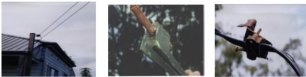
Figure 4 - Obsolete Aerial Service Cables (From Left to Right: Open Wire Service Cable, Red Lead Service Cable, Black Webbed PVC)
