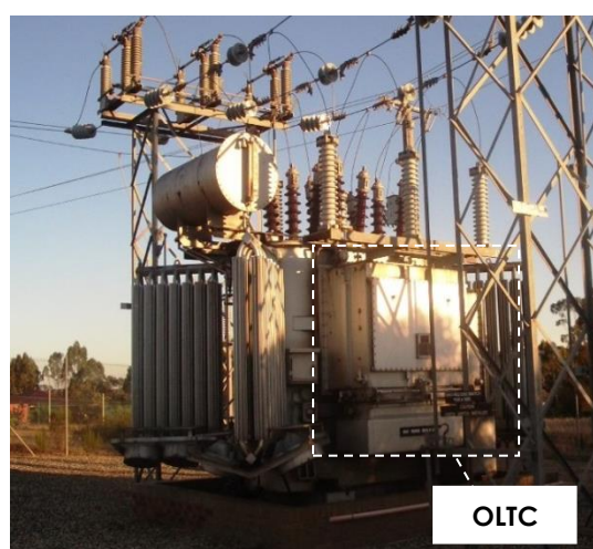
Figure 2: Typical Station Voltage Regulator with OLTC
