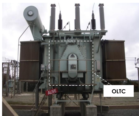
Figure 1: Typical Zone Substation Power Transformer with OLTC
