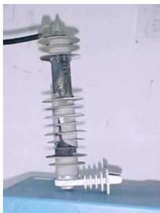
Figure 8 - Failure of Polymeric Surge Arrester Housing
