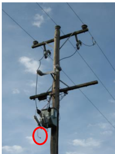
Figure 7 - Operation of an Earth Lead Disconnect
