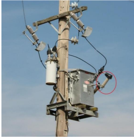
Figure 3- Polymer housed surge arrester fitted to an isolating transformer
