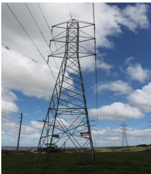
Figure 1: Typical 132kV tower.
