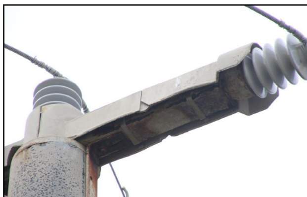
Figure 15 - Steel Crossarm rusting under an animal cover
