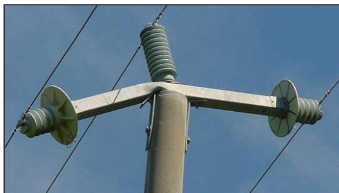
Figure 16 - Steel Crossarm Bending Failure
