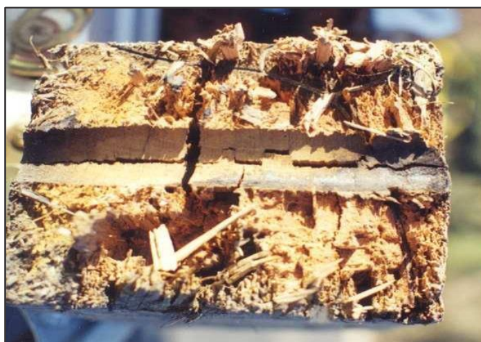
Figure 17 - Wood Crossarm Fracture
