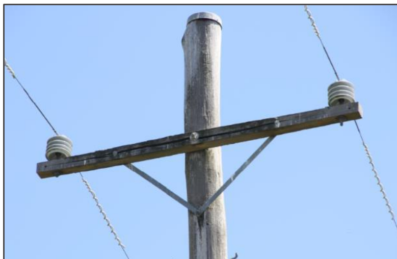
Figure 18 - Wood Crossarm Fracture at kingbolt
