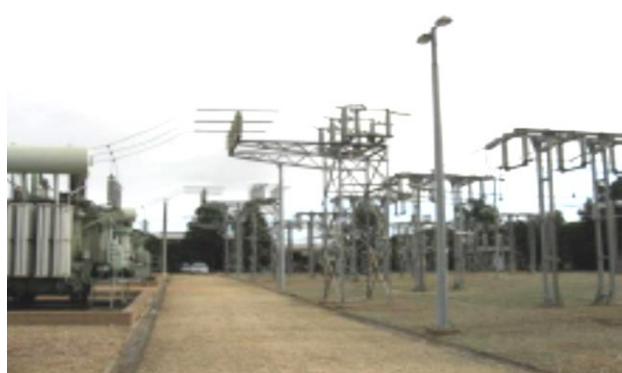
Figure 11 - Switchyard Lighting at Sale zone substation (SLE)
