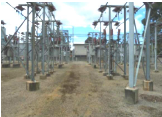
Figure 9 - Unsurfaced Switchyard surface at Watsonia zone substation (WT)
