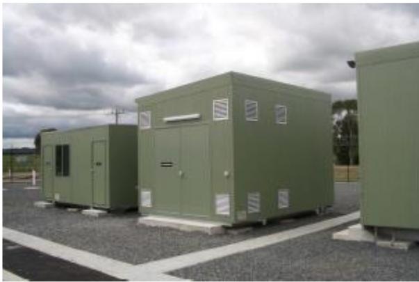
Figure 3 - Prefabricated buildings at Lysterfield zone substation (LYD)
