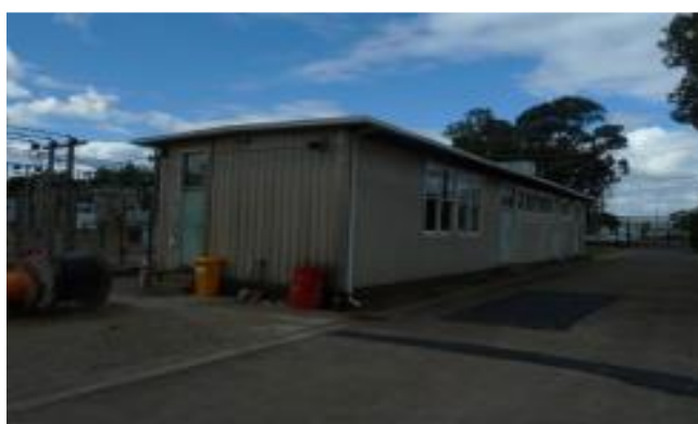
Figure 5 - ACM panels on a Control Building at Thomastown zone substation (TT)
