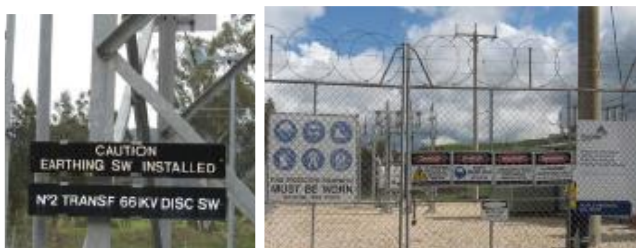
Figure 13 - Operational nameplates at Mount Beauty zone substation (MBY) and Perimeter and Gate Signage at Merrijig zone substation (MJG)
