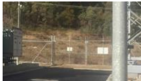
Figure 8b - Security fence & gate at Mt. Beauty zone substation (MBY), after augmentation
