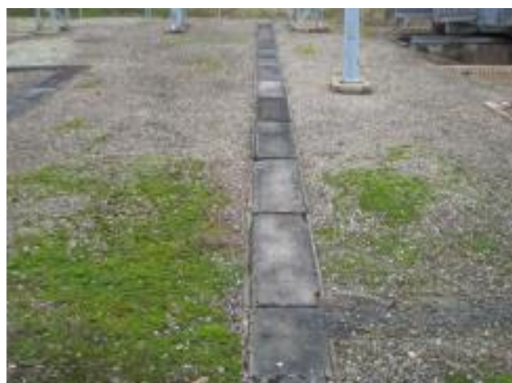
Figure 12 - Cable trench and cover lids at Mount Beauty zone substation (MBY)
