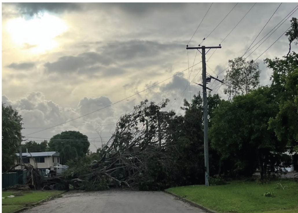
Figure 2: Fallen vegetation bringing down powerlines
