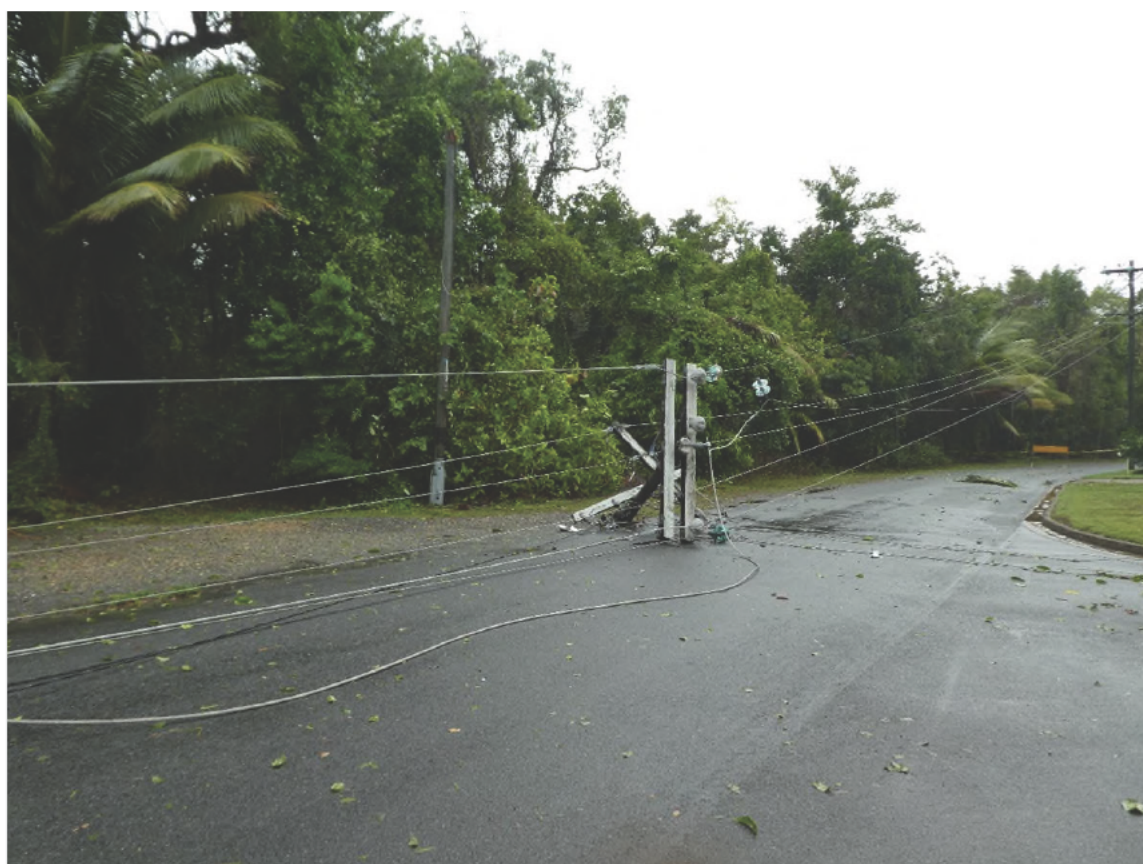
Figure 3: Broken HV Pole in Port Douglas
