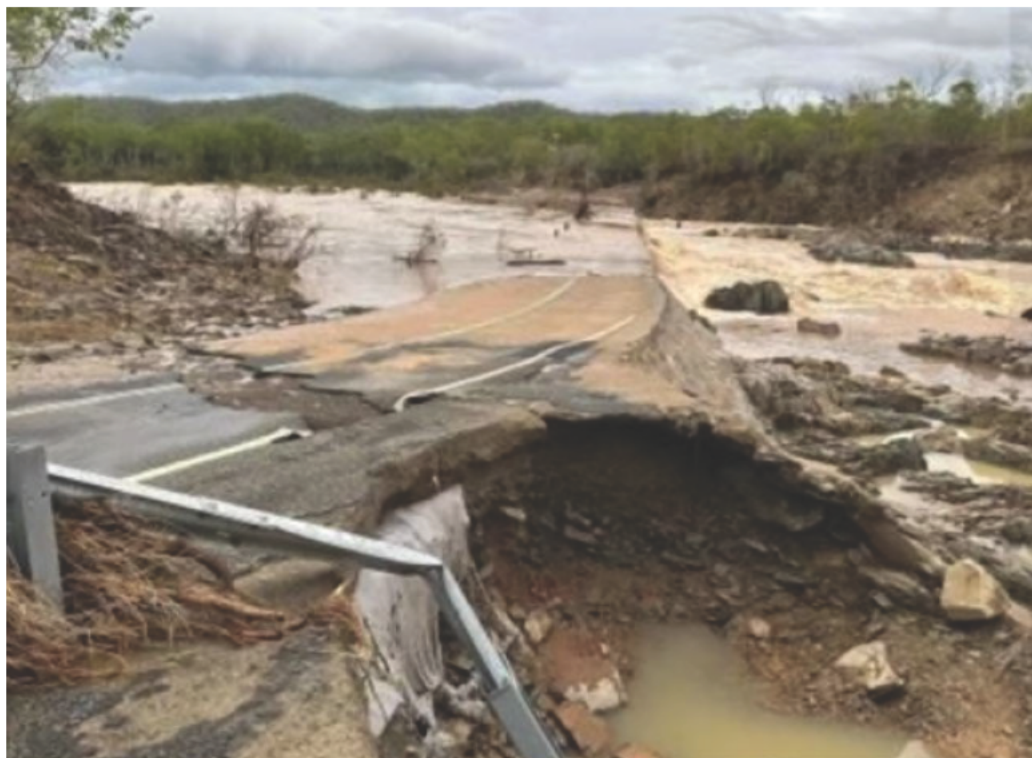
Figure 5: Road damage and flooding in Cooktown
