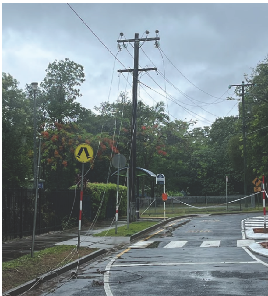
Figure 2: Network damage and fallen powerlines in Cairns
