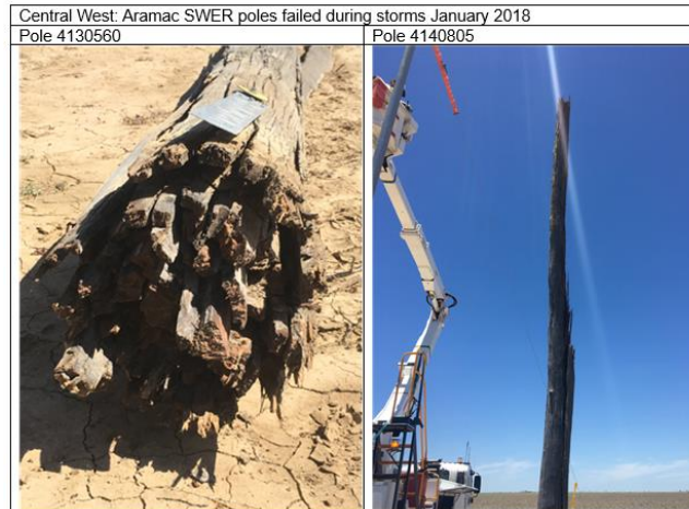
Figure 9 : Examples of 3kN unassisted pole failures
