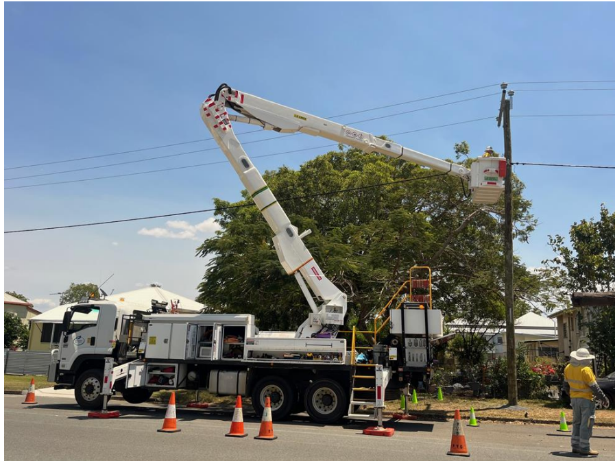
Figure 1: Example EWP in operation
