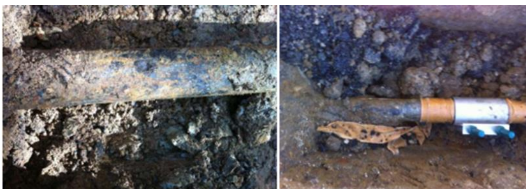
Figure 1-1&2: Examples of corroded cast iron mains and a repair clamp used throughout JGN
