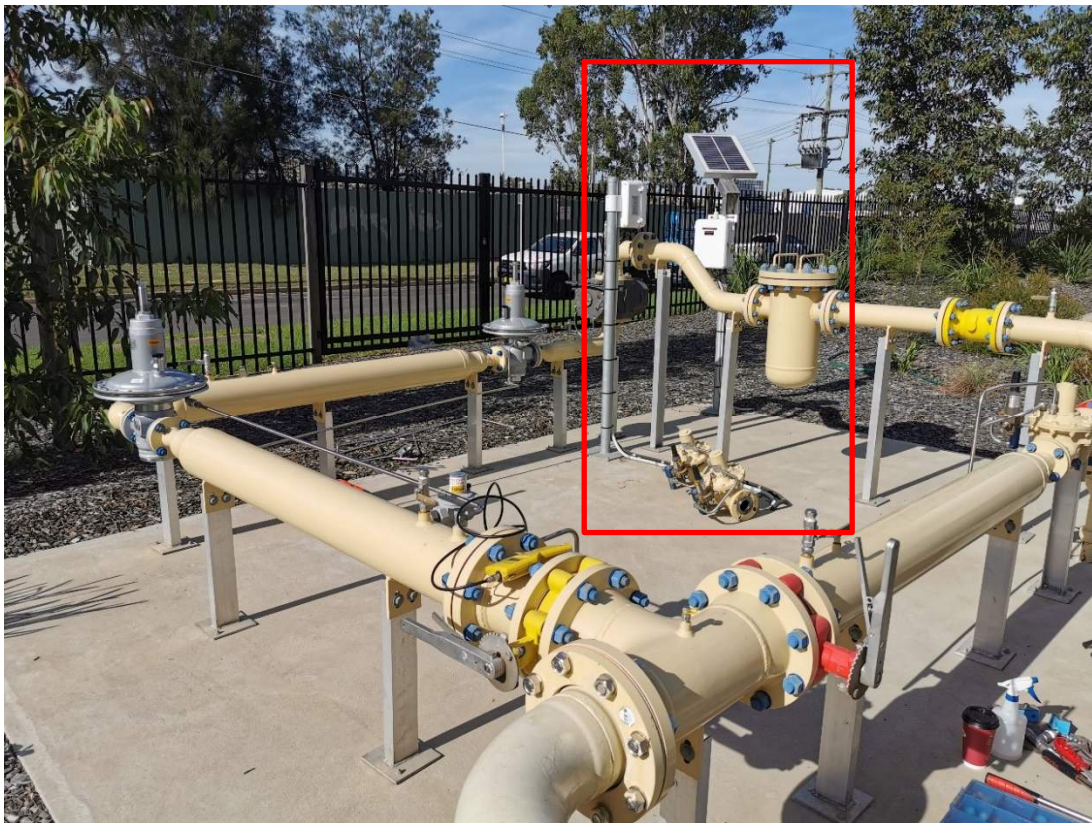
Figure 1: A typical Metretek system installed for a Demand Meter Set
