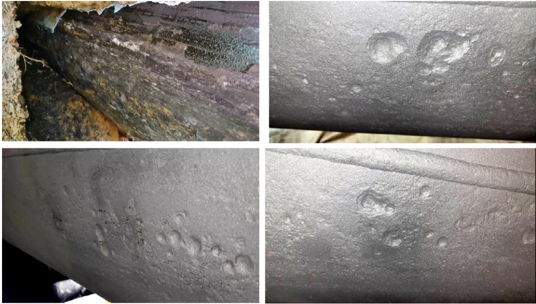
Figure 4: Corrosion Anomalies found on SPM (HP-Lid) - ILI
