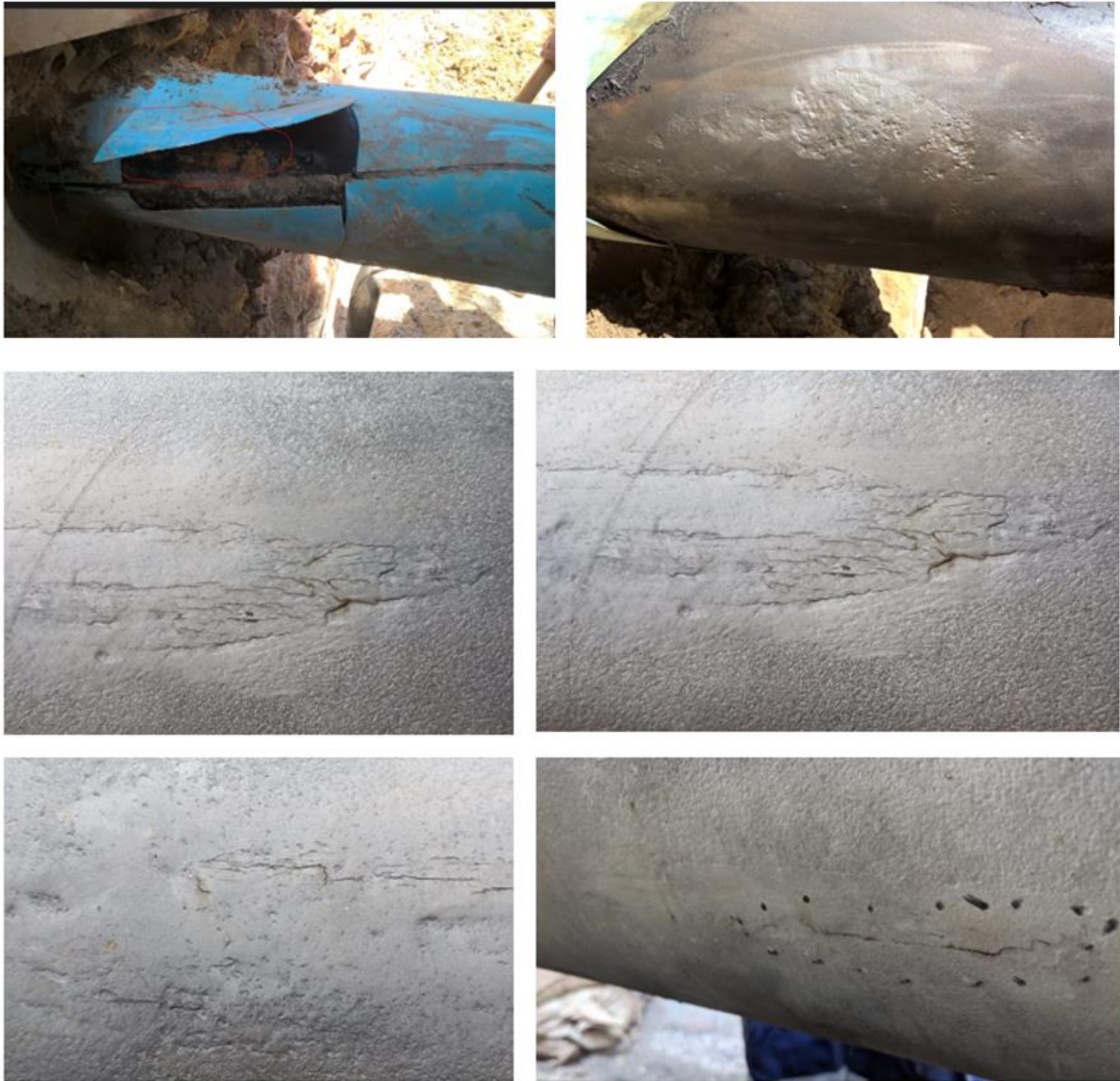
Figure 5: Coating Defect, Corrosion and Crack Like Features found on SPM
