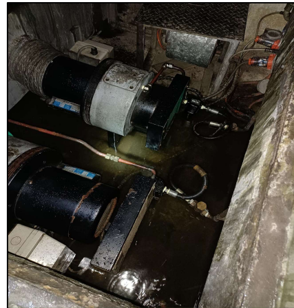
Figure 7 : Pit flooded during call out
