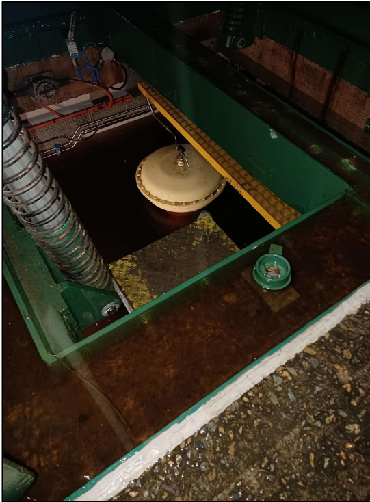
Figure 3 : Pit flooded during call out
