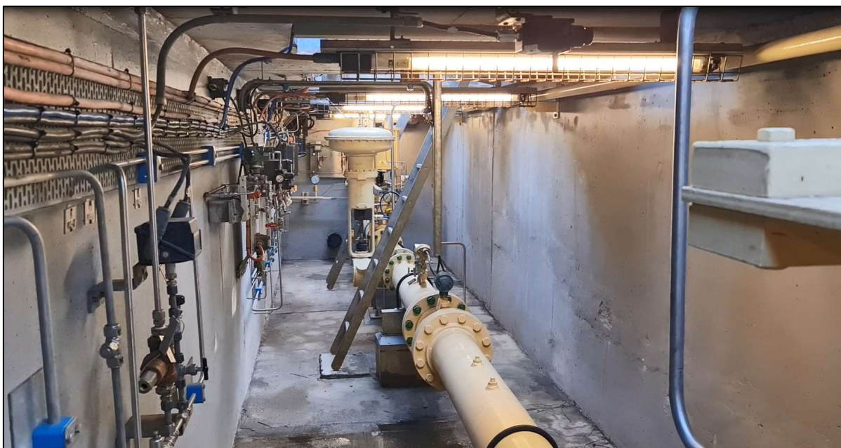
Figure 2 : Duty Run of Flemington PRS within a dry pit.
