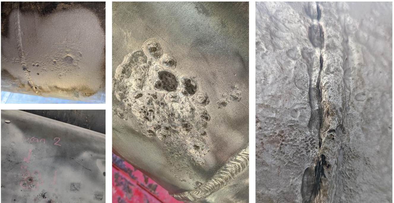
Figure 3: Corrosion Anomalies found on Licence 3, 7, 8a & 8b - ILI
