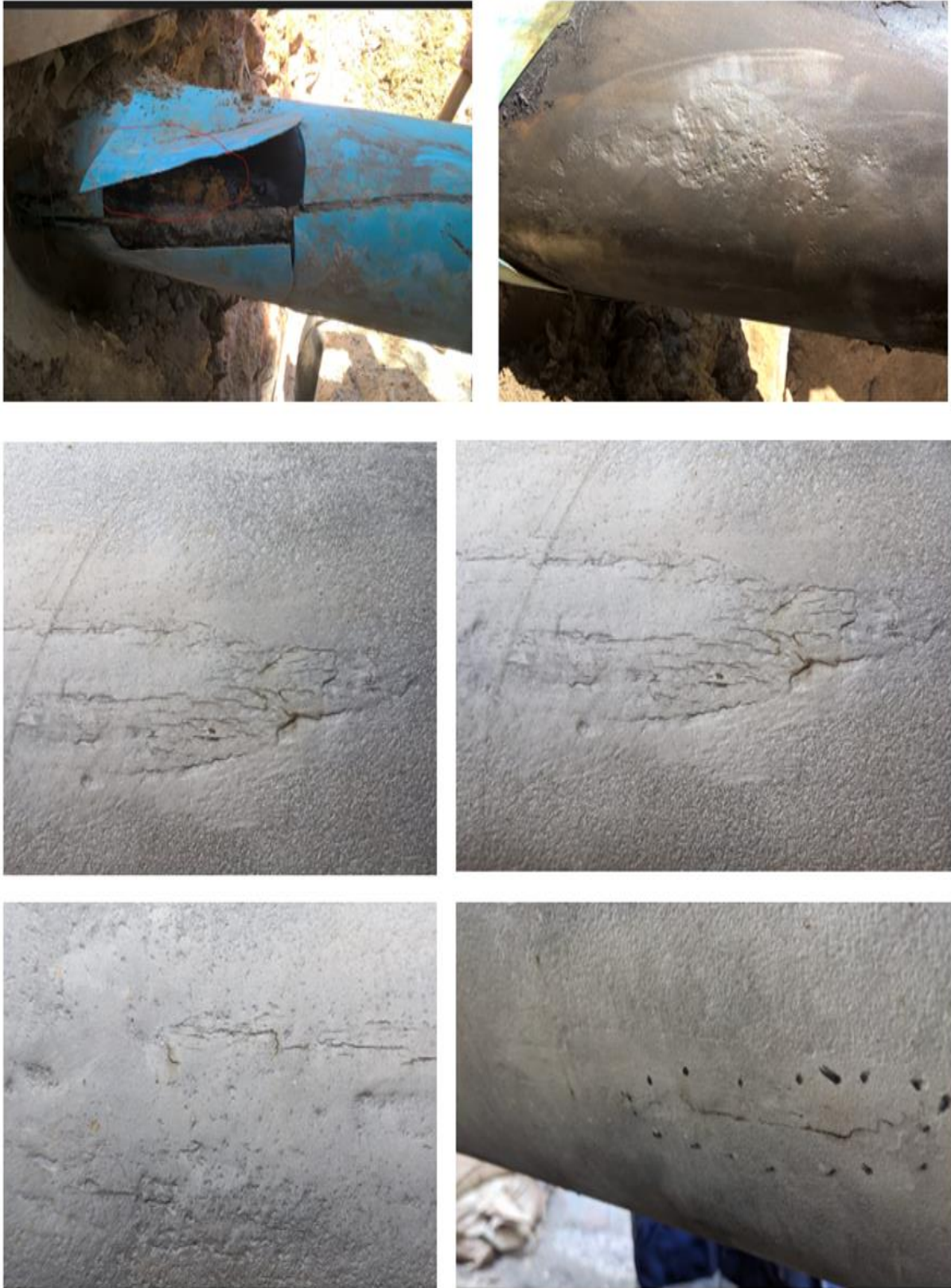
Figure 5: Coating Defect, Corrosion and Crack Like Features found on SPM
