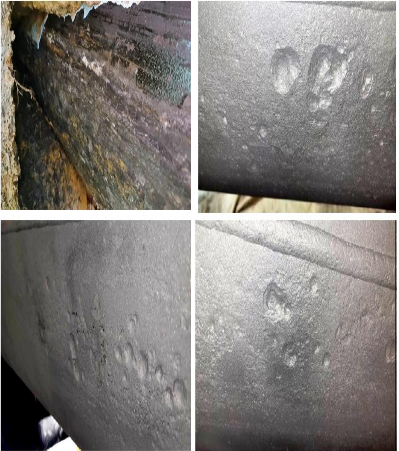
Figure 4: Corrosion Anomalies found on SPM (HP-Lid) - ILI
