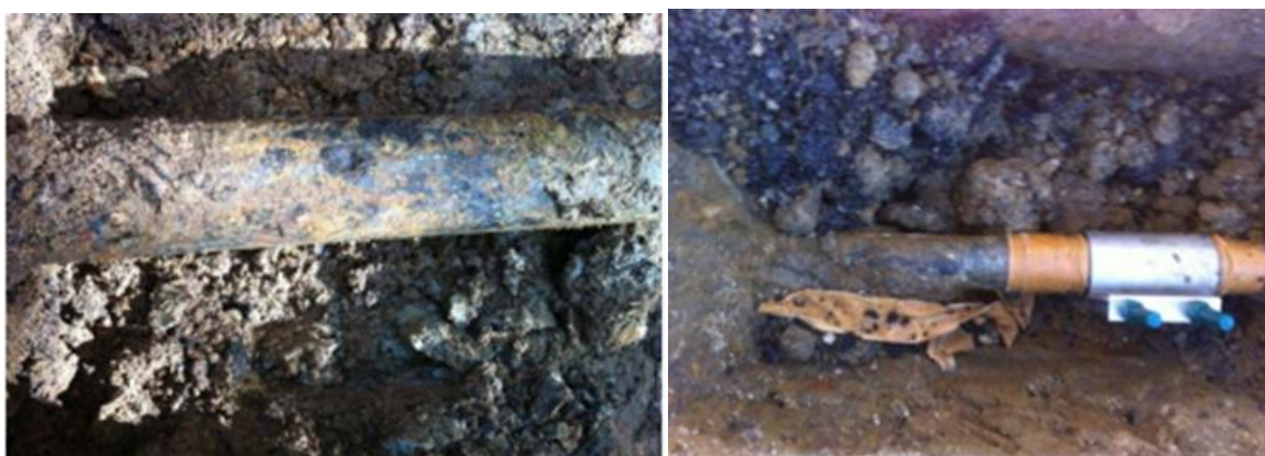
Figure 1 & 2: Examples of corroded cast iron mains and a repair clamp used throughout JGN
