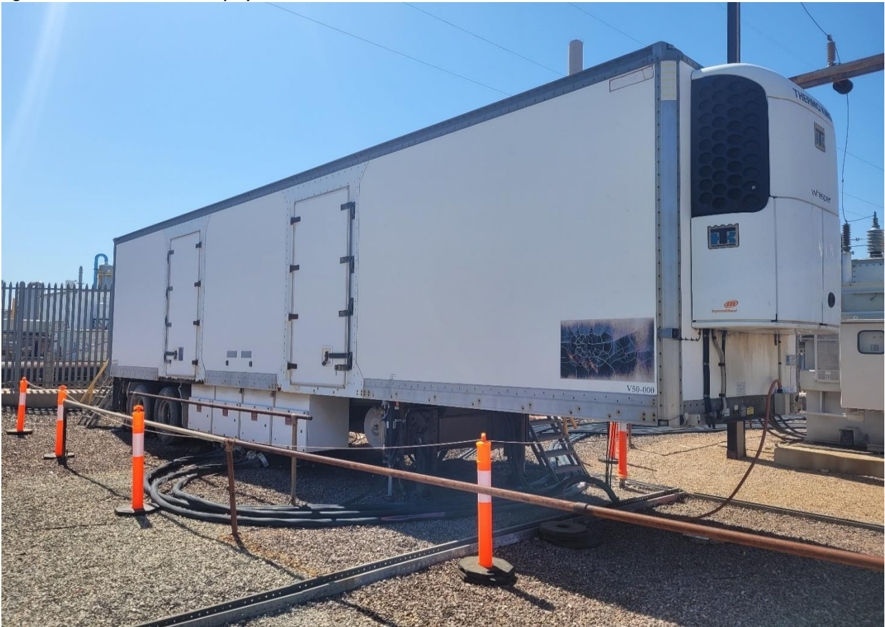
Figure 2: Mobile Switchboard deployed at Port Pirie
