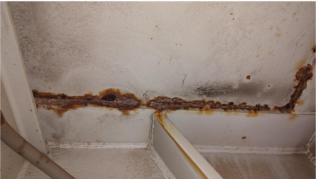
Figure 3: Visible corrosion between chassis top flange and floor on Mobile Substation
