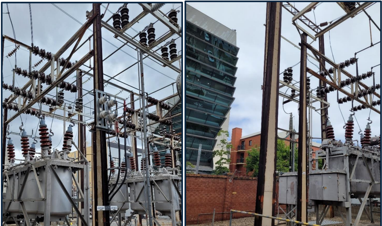
Figure 2: Bulk oil CBs below disconnectors (Left), and close proximity to CBD Street (Right)
