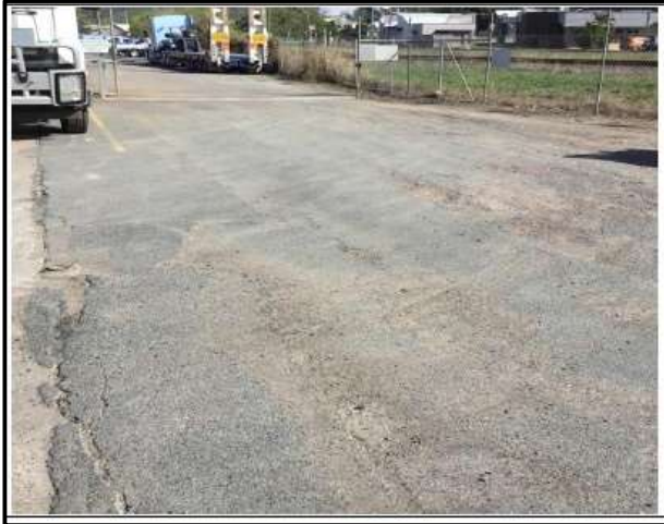
Yard Surface – Entire pavement failed
