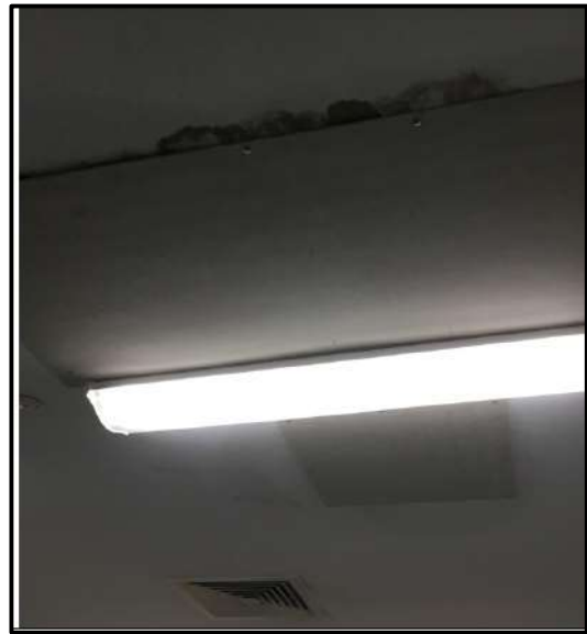
Building A – Ceiling water damage
