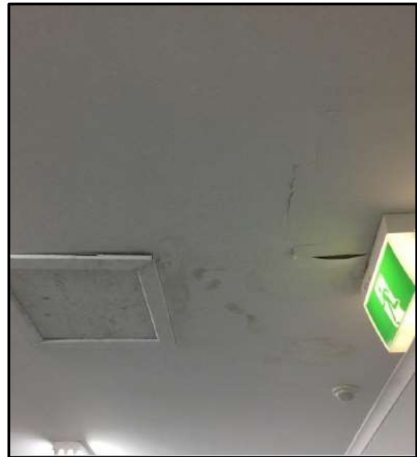
Building A – Water damaged ceiling
