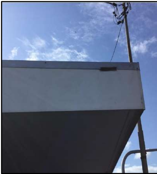
Building A – Box gutter overflow
