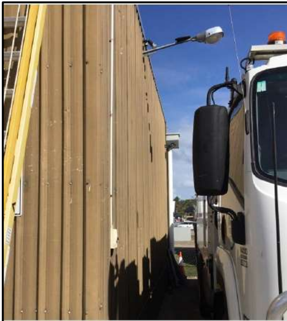
Building B – Aged wall sheets & flashing
