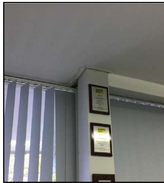
Building A – Internal water ducting, ceiling & floor damage
