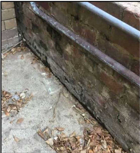
Retaining Wall – Water run-off causing failure
