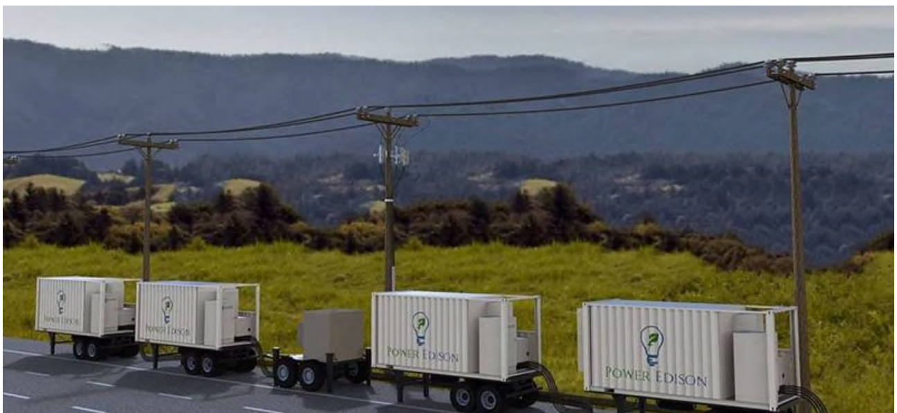
HV mobile battery units
