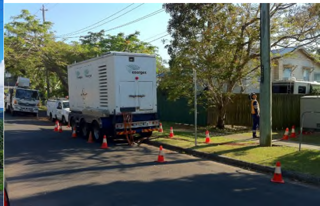
LV mobile generators
