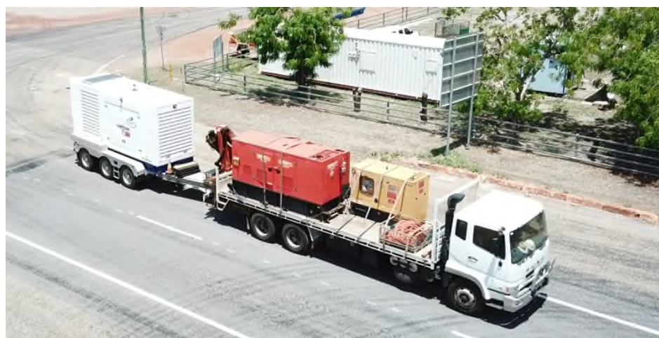
Figure 1 – Deployment of LV mobile generator
