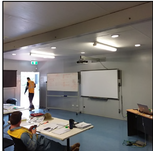
Block 9 – Internals (trip hazards throughout, inefficient lighting & acoustics for training, temporary furniture)
