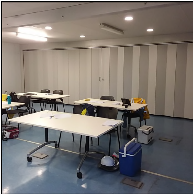
Block 9 – Internals (trip hazards throughout, inefficient lighting & acoustics for training, curtain wall)
