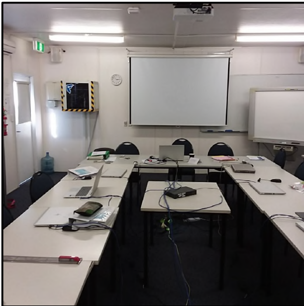
Block 8 – Internals (note: constrained space for training, sagging ceiling)
