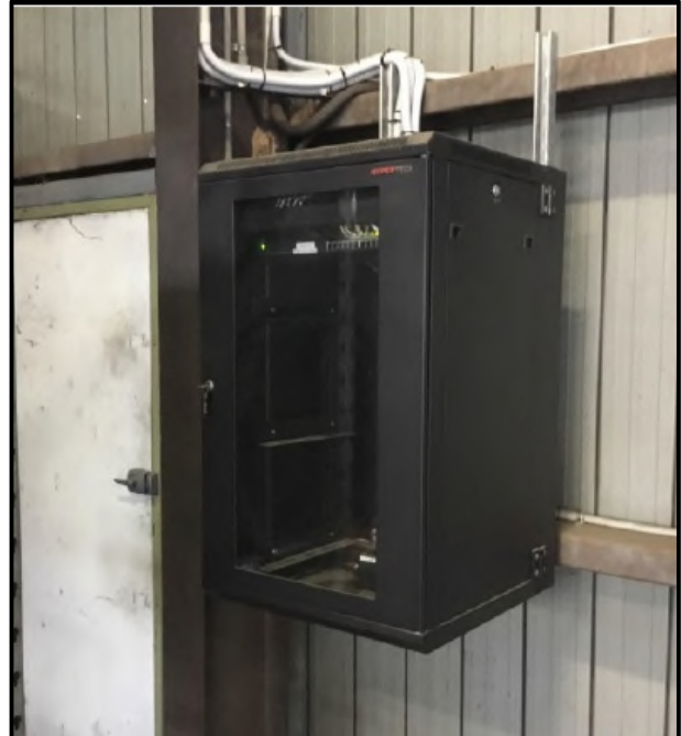
Building B – Data/Comms equipment in open warehouse
