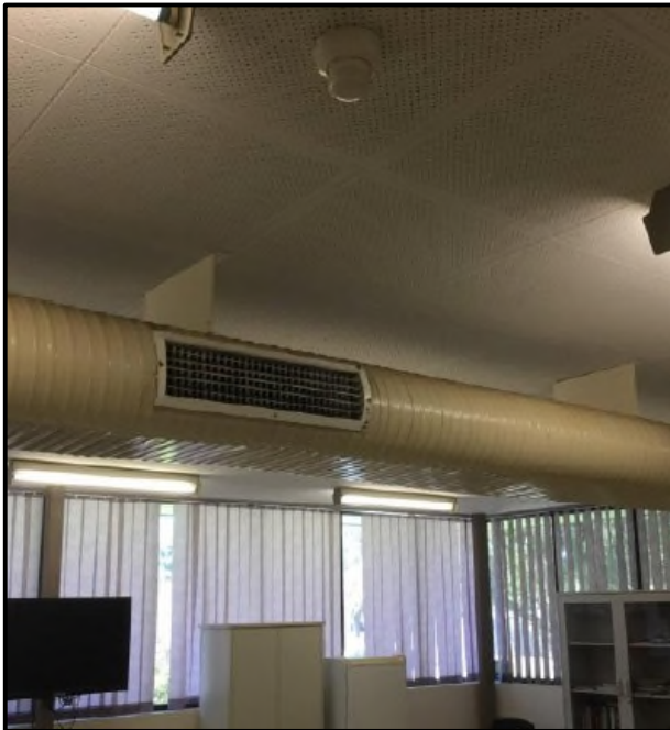
Building A – A/C ducts run internally, noise & dust transfer
