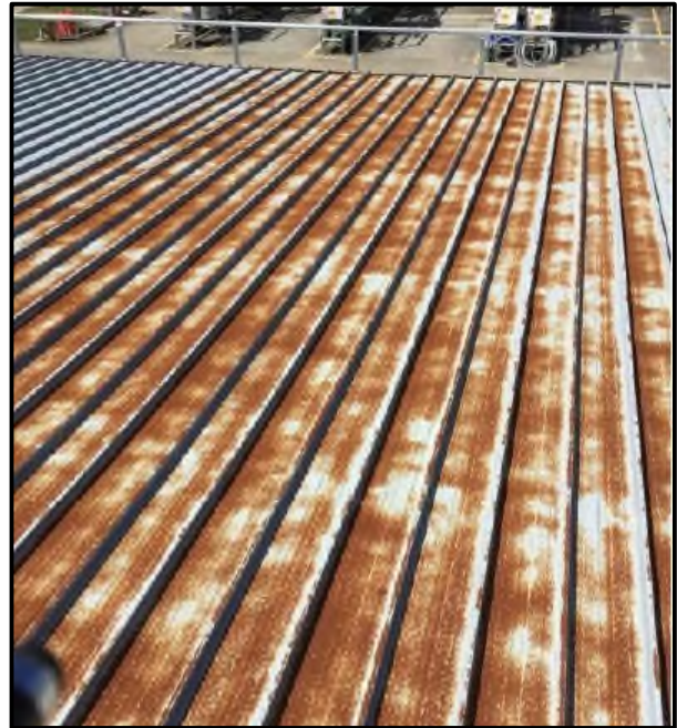
Building B - Roof deterioration
