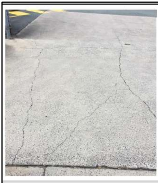
Yard Surface – Concrete cracking
