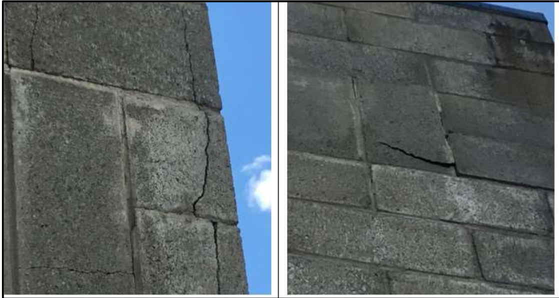
High-level storage – Masonry cracking
