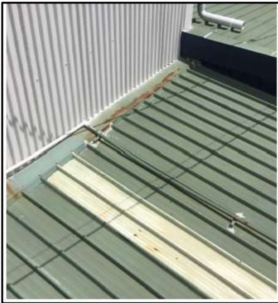
Admin – Roof sheet corrosion and flashing failure
