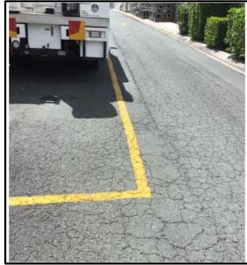
Yard Surface – Bitumen crocodile cracking
