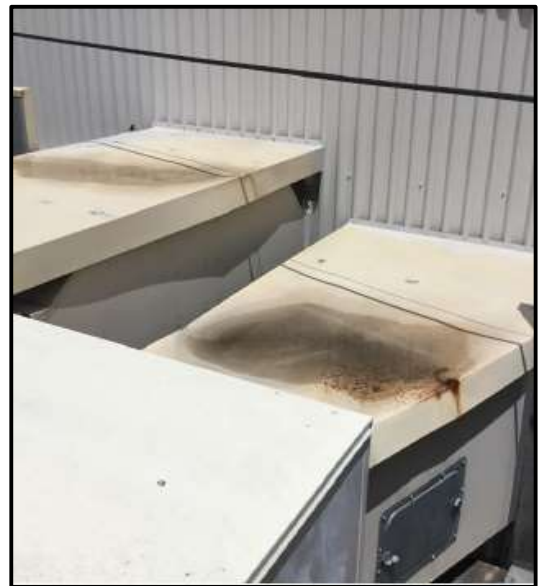
Admin – A/C plant protection failing
