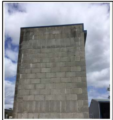
High-level storage – Considered unstable, severe cracking, foundation concerns
