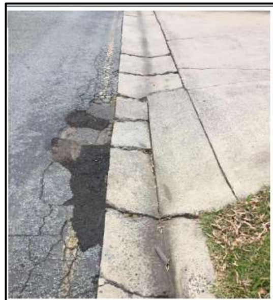
Yard Surface – cracking along joints
