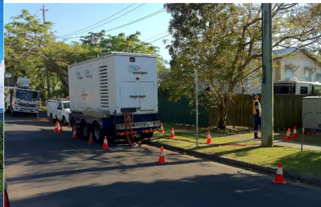
LV mobile generators
