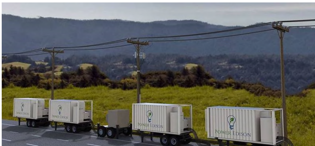
HV mobile battery units
