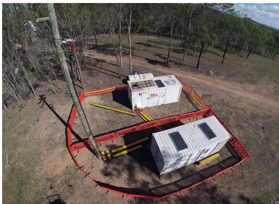
Figure 2 – Pegasus mobile generator at the site
