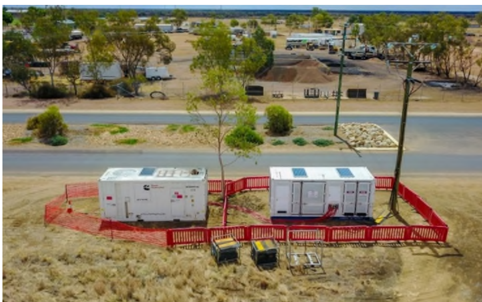
Ergon's HV Pegasus mobile generator
