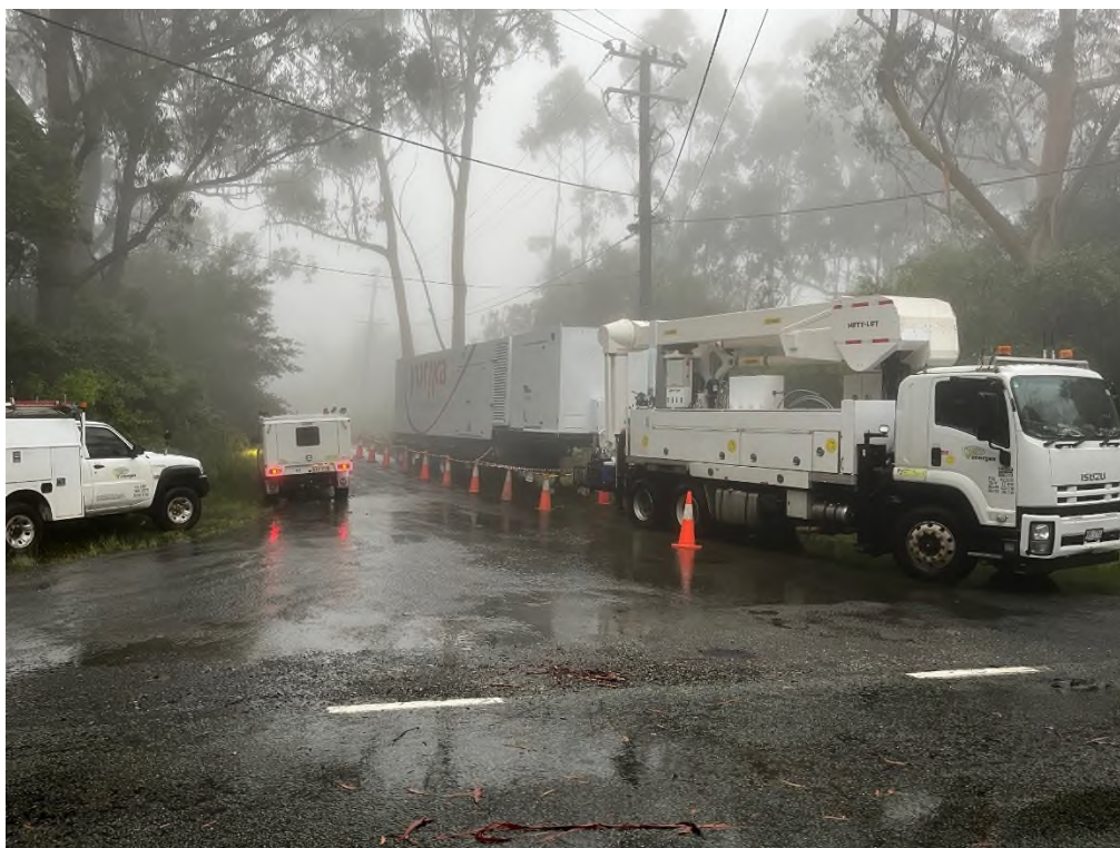
Use of mobile generators during the storm restoration on the Gold Coast (December 2023)
